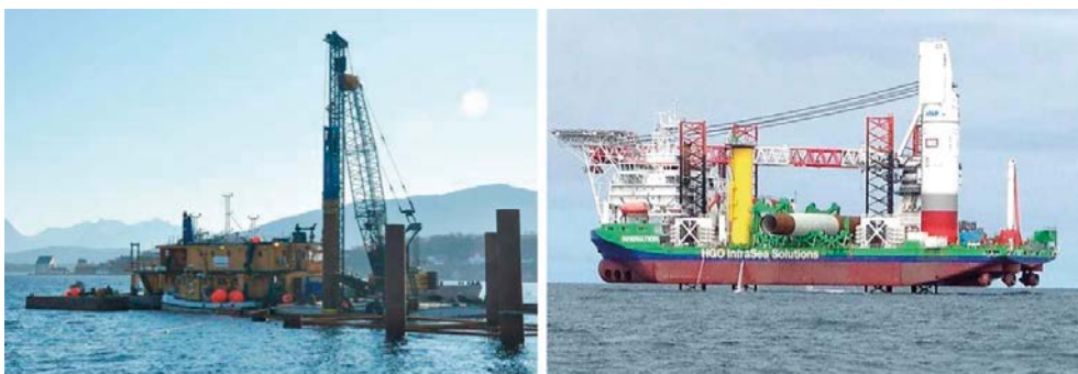
Figure 7. Left: Pile driving of a port structure in Ålseund, Norway (Photo: Mathias Andersson, FOI). Right: A pile driving ship in the German North Sea prepares the installation of an offshore wind turbine foundation (Photo: Markus Linné, FOI).
